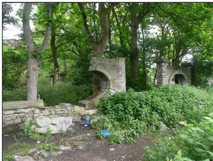
Illus. 30: West part of the east-west wall showing deterioration caused by partial collapse since 2006.
