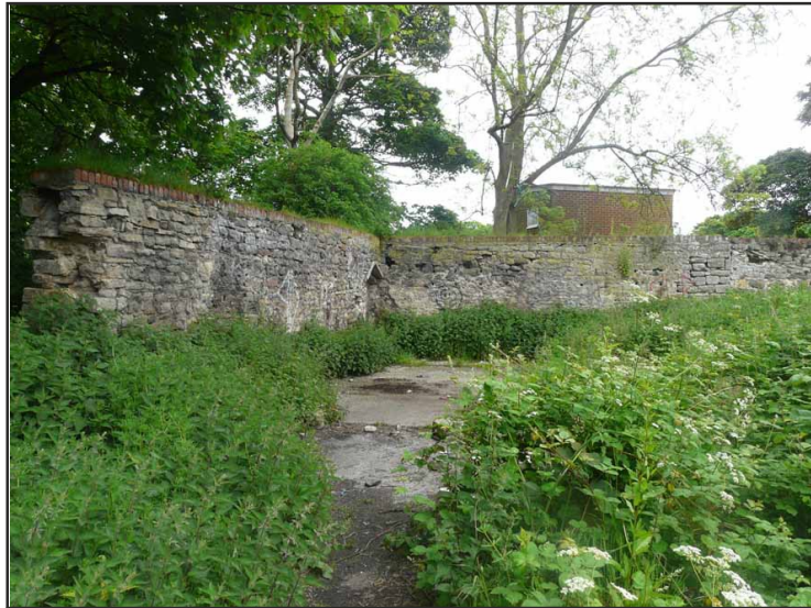
Illus. 22: The surviving north wall of Whitburn Tithe Barn (left), forming an east-west dividing wall within the assessment site with possibly-contemporary east site boundary wall to right of view.
