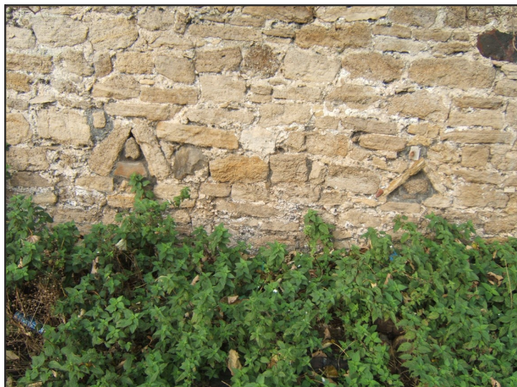
Illus. 24: Vents in the surviving north wall of Whitburn Tithe Barn, south-facing elevation.
