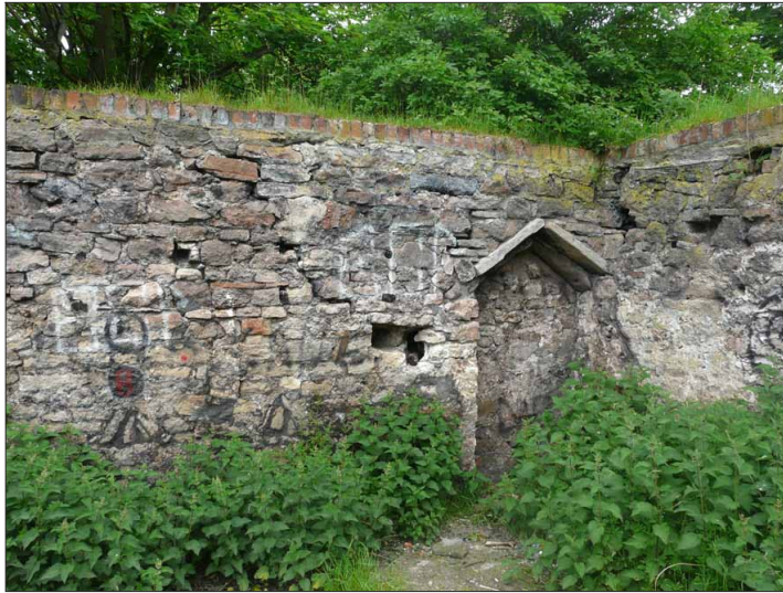
Illus. 25: Blocked door at the east end of the north wall of the former tithe barn.
