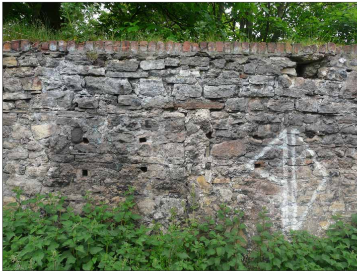
Illus. 26: View from the south of a blocked doorway at the east end of the tithe barn north wall.
