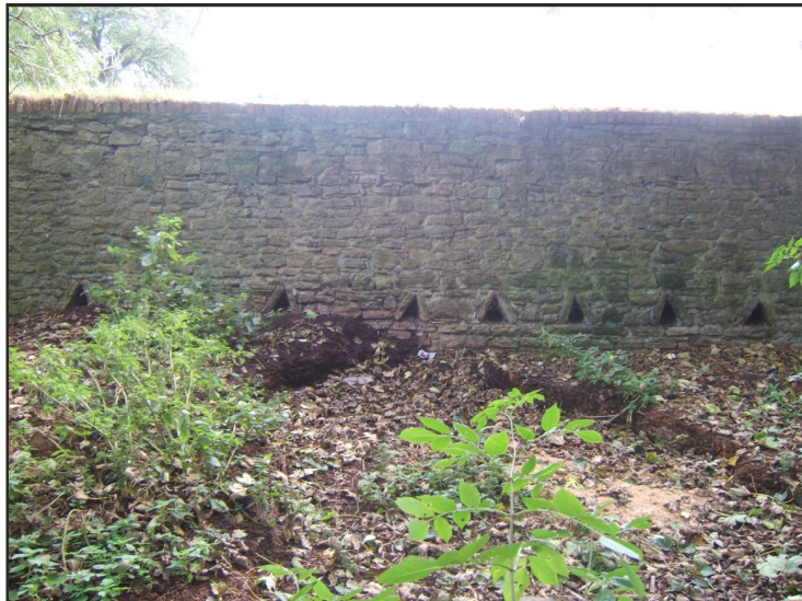
Illus. 23: The surviving north wall of Whitburn Tithe Barn viewed from the north side.
